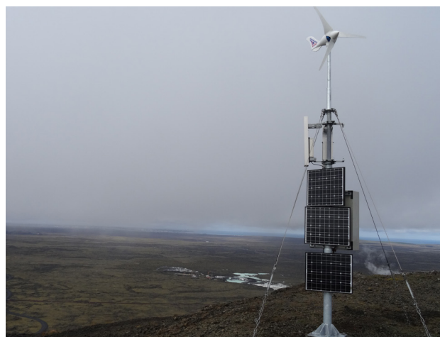
Seismic Monitoring System
